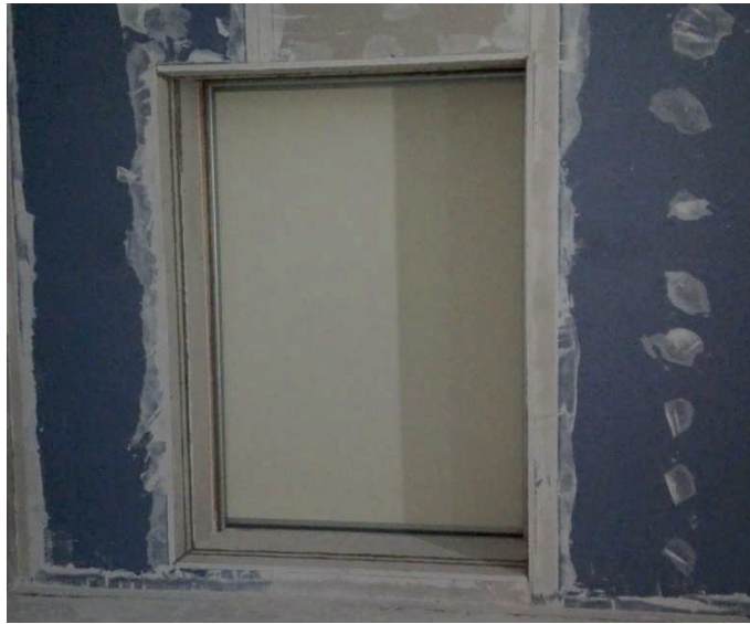
Figure 1: Emitting room side
